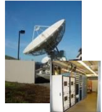
6 Ground Earth Stations
