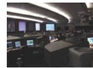
2 Operational Control Centers
