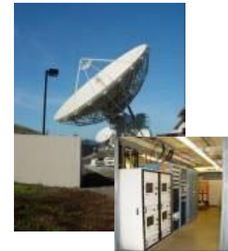
6 Ground Earth Stations
