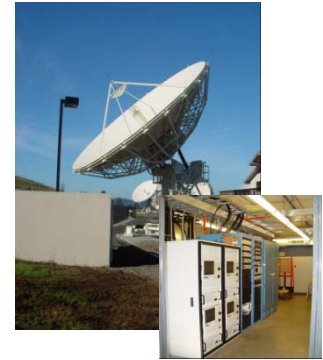
4 Ground Earth Stations
