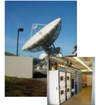
4 Ground Earth Stations
